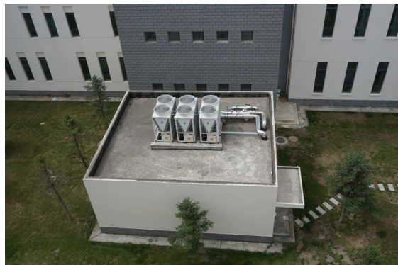
热源机房及低温型风冷热泵
